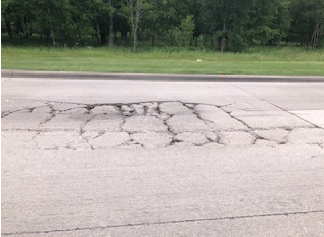
Example of Needed Repair #4. Via Toscana near the bridge
