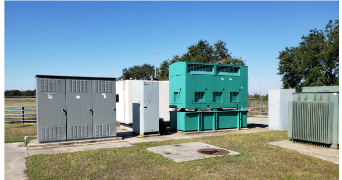
LNVA, FEMA Mitigation
